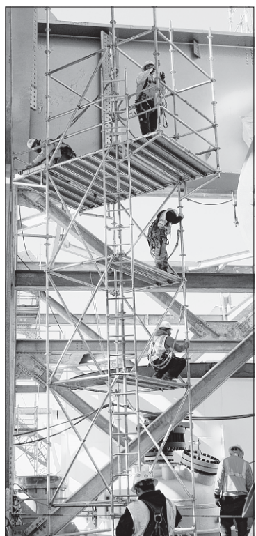
Workers erect a scaffold at Mississippi Power's Kemper County energy facility near DeKalb, Miss.
