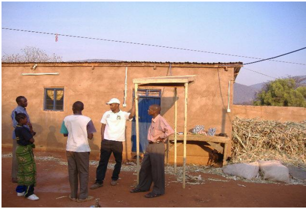
Figure 7b: Wrong wire run length, size and module mounted on wooden poles.
