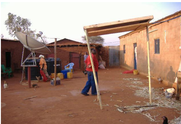
Figure 7c: Wrong wire run length, size and module mounted on wooden poles.
