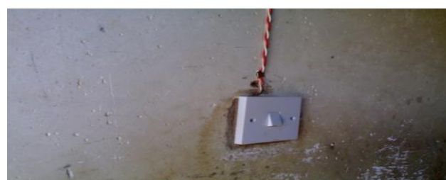
Figure 7a: Wrong cable size used for installation.
