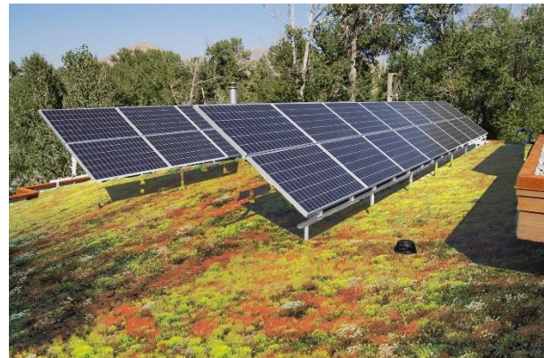
Figure 1. Integration of PV panels on the green roof.
