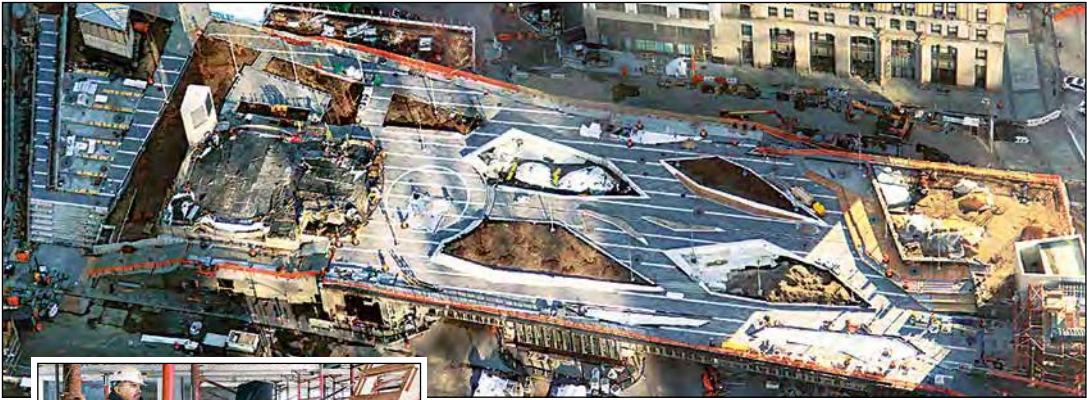
The site in January 2016 shows work being done under the base of the church.
