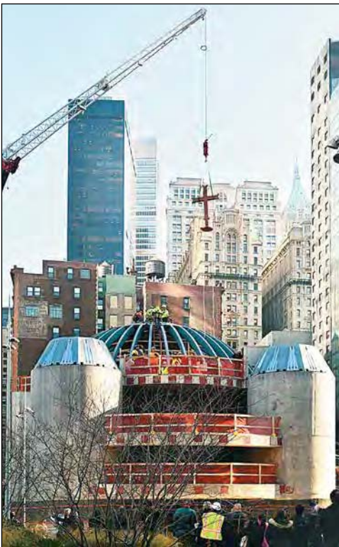
A large crane lifts the 6 ft. cross high above the construction site and onto the dome.
