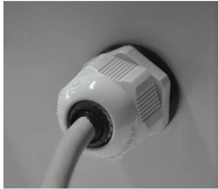
AC power cable running through cable gland with plastic nut ( ground wires are not visible from this perspective )
