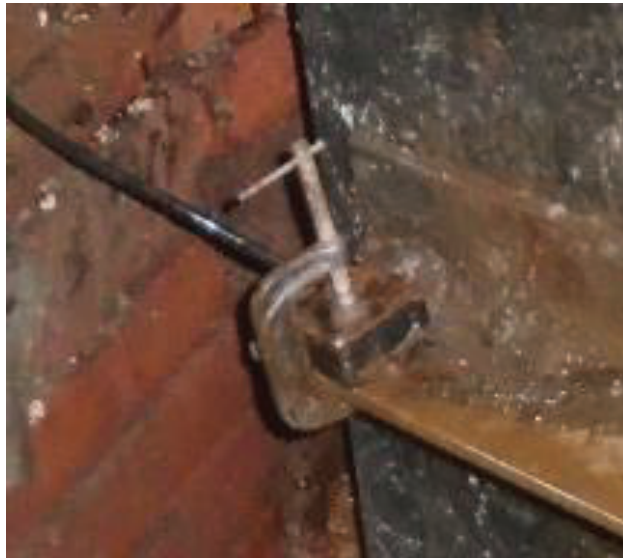
Inclinometer attached using a Stainless Steel Clamp
