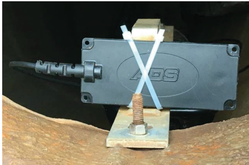
In-Manhole Antenna Installed to Mounting Bar with Cable Tie
