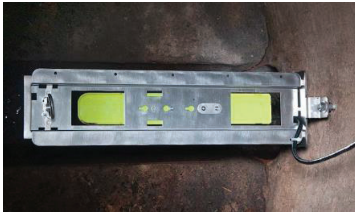
Installed Sensor Bracket on Wall Mount Bracket
