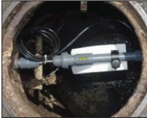
Long Range Sensor Fully Installed
