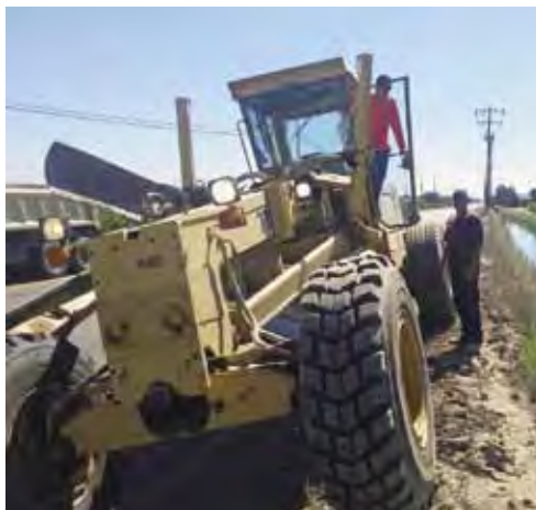
Former Fresno Irrigation District negotiating team member/Scraper Operator Robert Metzler and member Rod Thatcher work on a canal.
