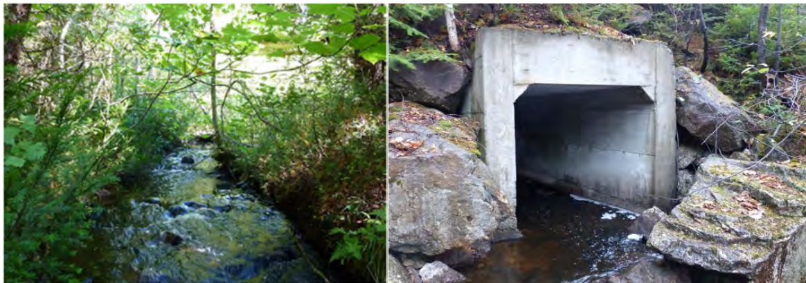
Figure 2. A (left). The brook downstream from the culvert; B (right). The culvert under the road 172. Photos by Jacques Desbiens.
