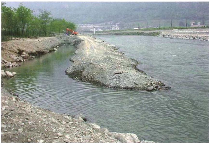
Fig. 9: Experimental restoration site on the River Adige near Lana in construction (2003). (Foto: Irene Schatz)
